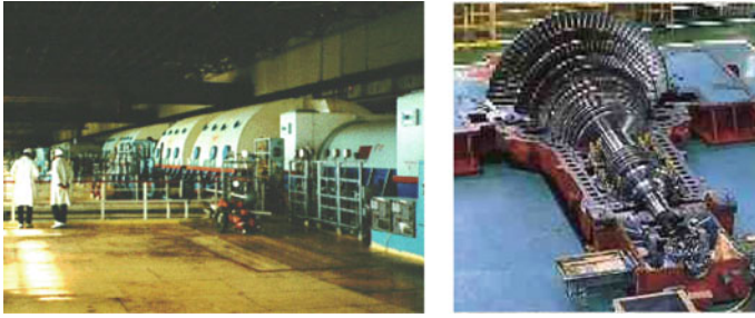
Fig. 5.18 Steam turbine generator unit
